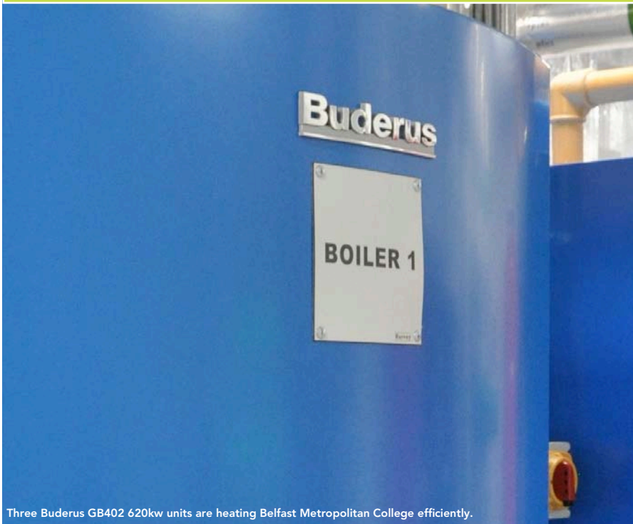
Three Buderus GB402 620kw units are heating Belfast Metropolitan College efficiently.
